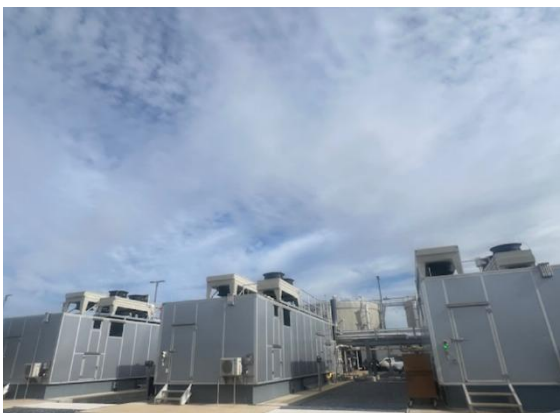
3 CHP's, 1.5 MW each
